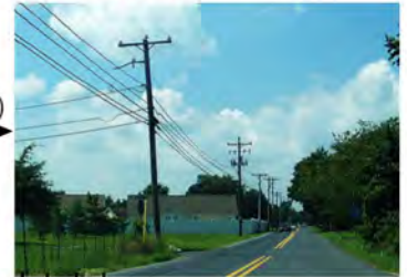
Medium & Low Voltage Distribution Line
