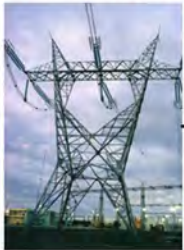
Extra High Voltage Transmission Line
