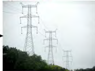
High Voltage Transmission Line
